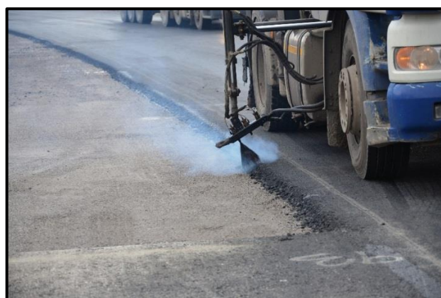
Figure 17: Sealing the vertical edge of a longitudinal joint with a hot binder
